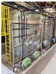
Perry Chemical Feed System
