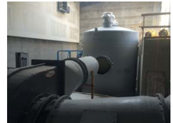
Perry B2 Unit with Mist Grease Filter, Fan and Ductwork
