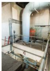
Odor Control Ductwork
