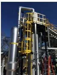
Left Photo: Perry Air Stripper / Degasifier in operation
