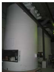
Right Photo: Perry 50,000 cfm Chemical Scrubber with pumps, controls, packing and feed pump. Installed in 2004
