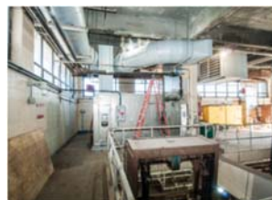
Waste Water Plant Odor Control Ductwork
